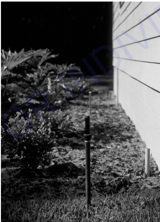
FIGURE A.17.1.8.1(b) Use of Low Volume Sprinklers in Organic Material. [1144:Figure A.4.2.4.1(b)]
